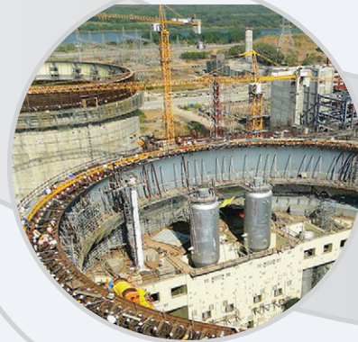
Main Plant Electrical Package for 2 x 700 MWe Kakrapar Nuclear Power Project
