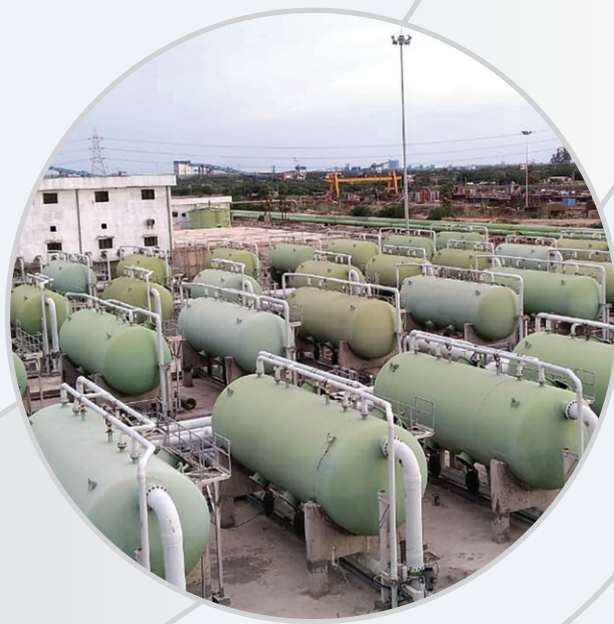
55 MLD Sea Water Desalination Plant at 800 MW Krishnapatnam Thermal Power Plant
